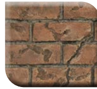
FIRE CRACKED BRICK
